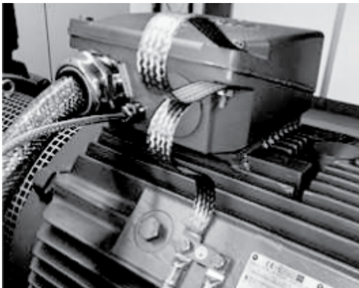
Illustration 17: Installation of EMC straps from the Terminal Box to the Motor Frame
