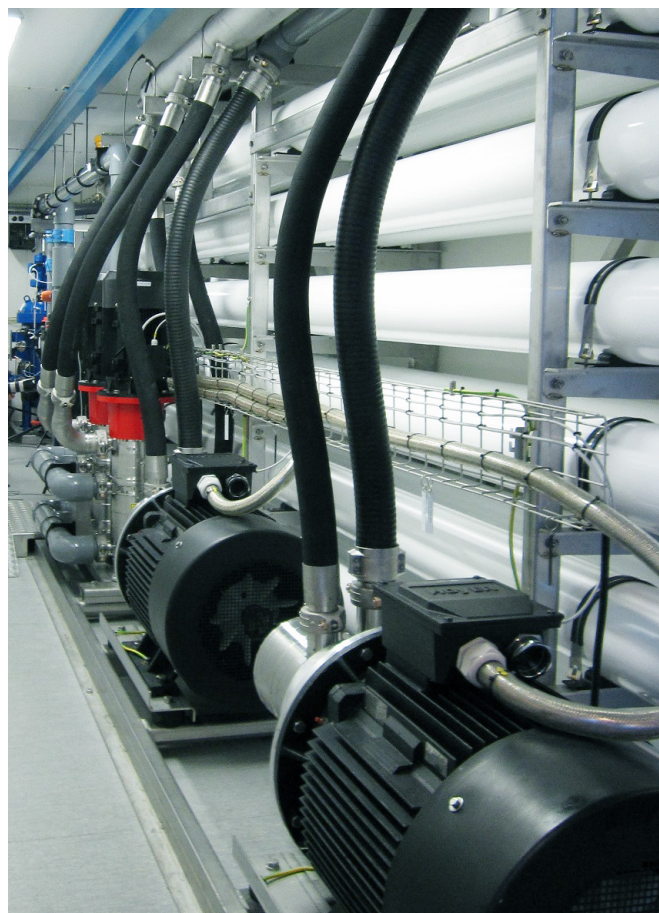
Containerized unit built with 2 APP 30 pumps and 2 iSave 40. Photo: Enwa Water Treatment.
